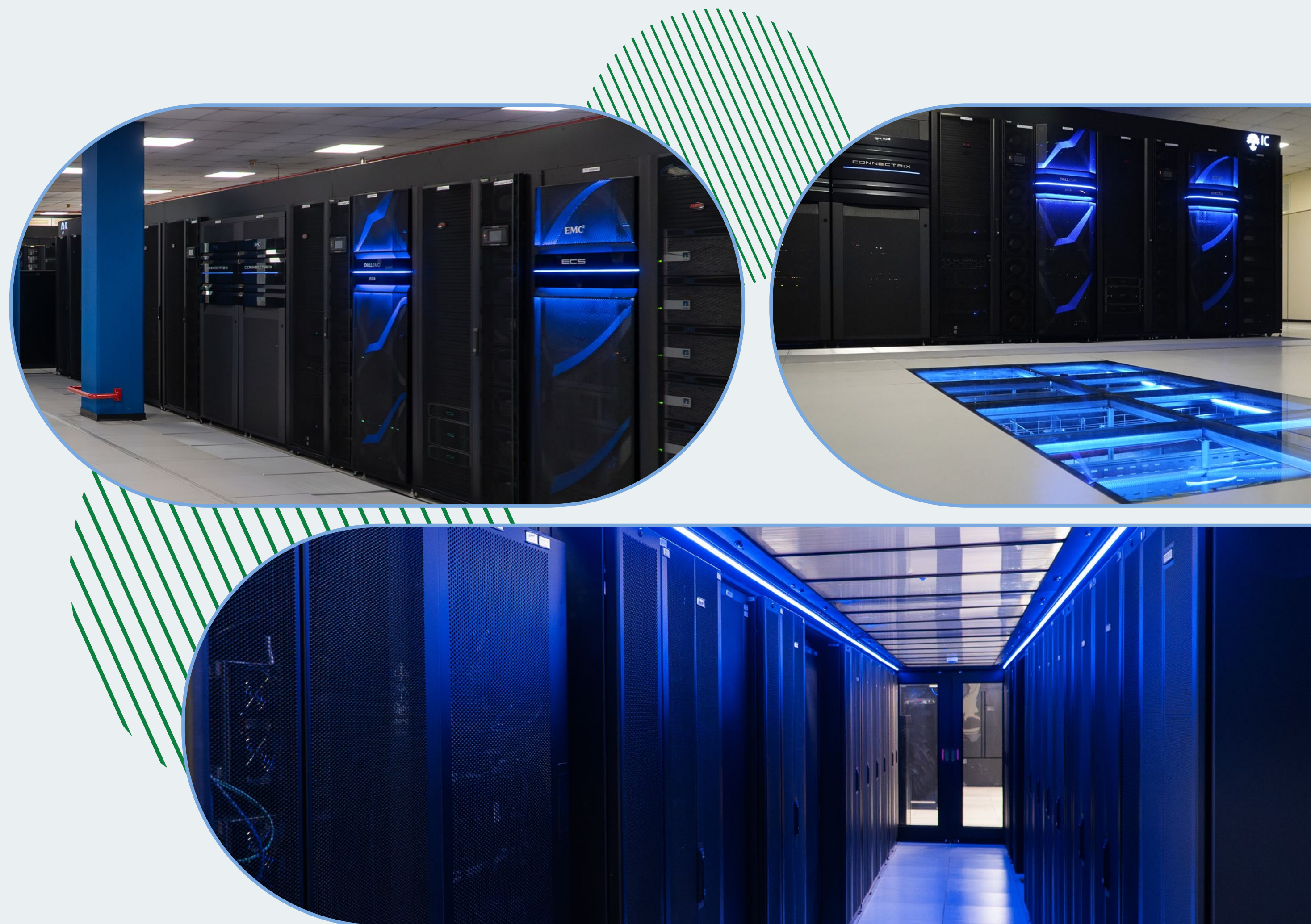
Data Center Padova
