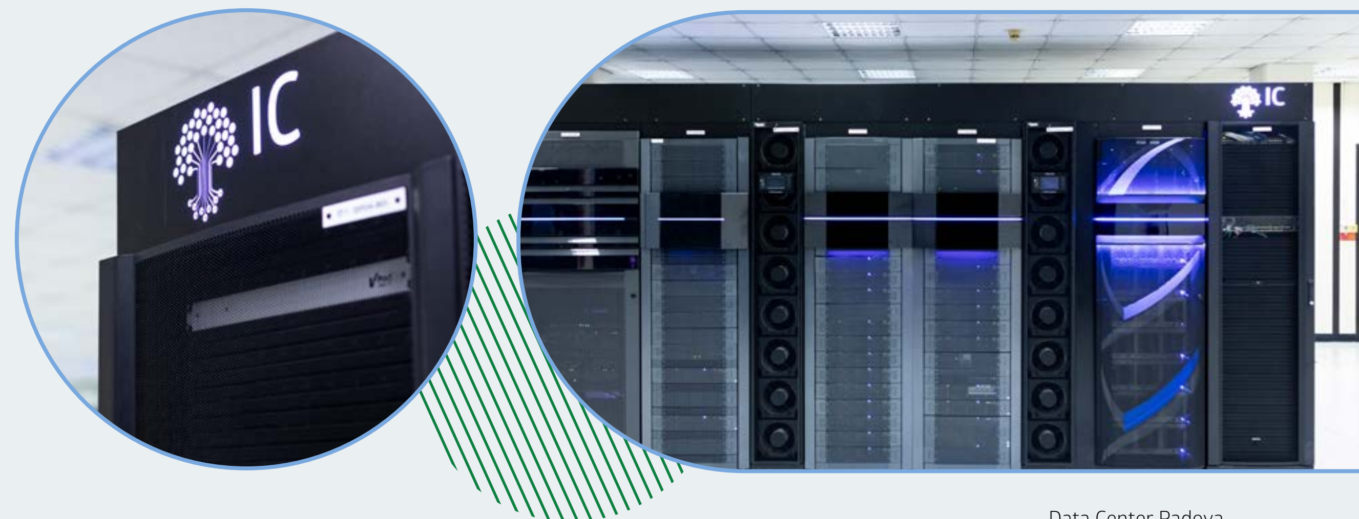
Data Center Padova
